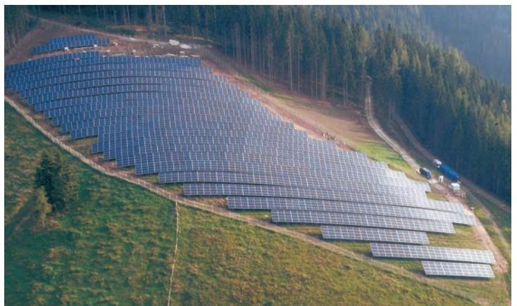
→ SOLARPARK KINDBERG, 1 MWP
