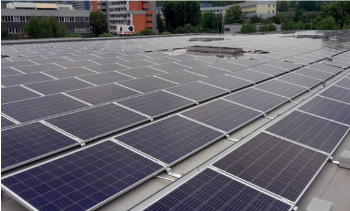
→ KNEIDINGER CENTER LINZ, LINZ STROM, 150 KWP
