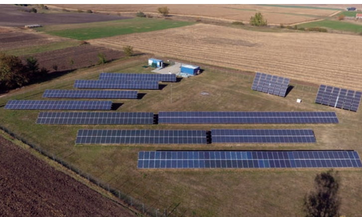
→ SOLARPARK NEWERGIES, UNGARN, 110 KWP
