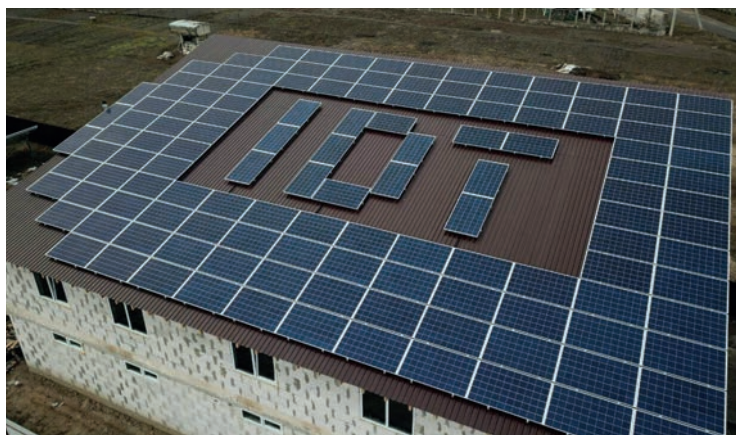
→ UTEM SOLAR, HOSTOMEL, UKRAINE, 36 KWP
