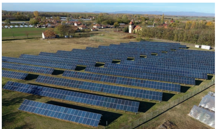
→ SOLARPARK NEWERGIES, UNGARN, 500 KWP
