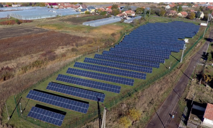
→ SOLARPARK NEWERGIES, UNGARN, 545 KWP
