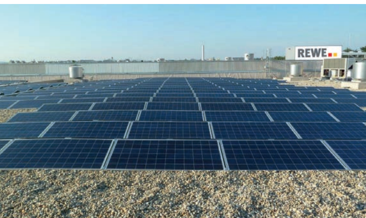
→ REWE INZERSDORF, 100 KWP
