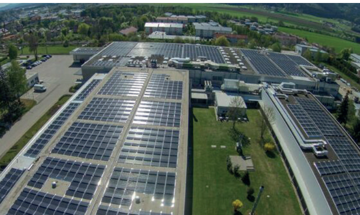
→ KÄRNTEN SOLAR, FLEXTRONIC, 1 MWP
