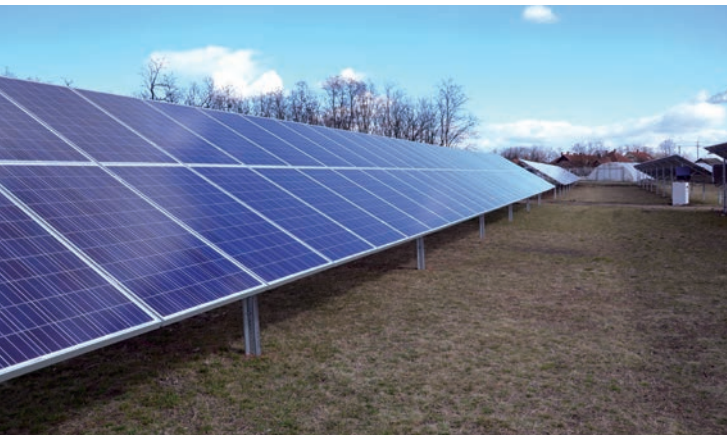
→ SOLARPARK NEWERGIES, UNGARN, 1 MWP
